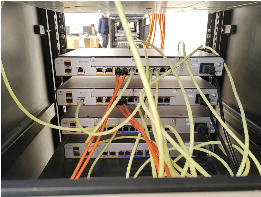
Figure 4: 机柜背面接线图
